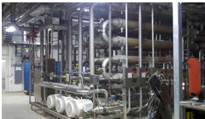
Picture 1. External AnMBR system with Berghof Membranes UF modules
