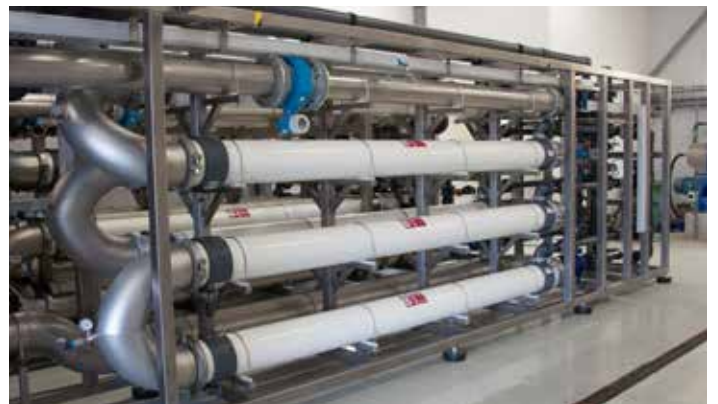
Picture 1. Photo of the B-SMART System installed at Holland Malt
