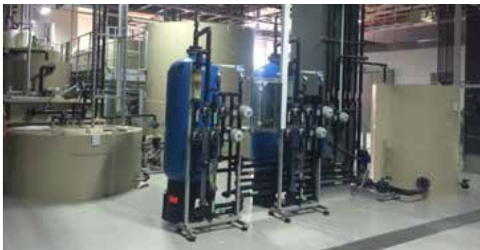
Picture 1. Physical chemical treatment plant
