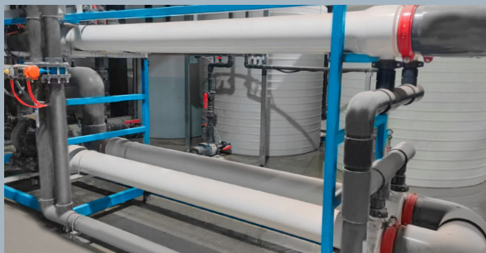
Figure 3. Tubular UF system in Huguan facility.
